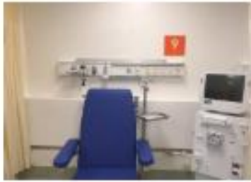
GCR Panel with American gases outlets and Chile / Brazil / Italy electric sockets
